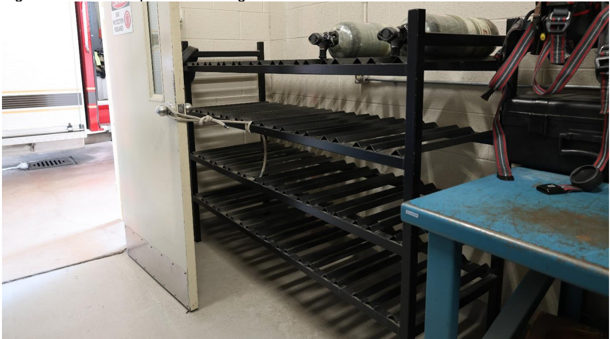
Figure 7 - SCBA Repair and Storage Room
